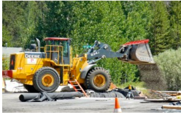
The Bijou erosion control project. Photo/LTN file
