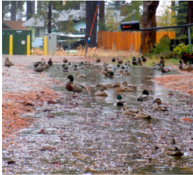
Some South Lake Tahoe streets have drainage issues every winter.
