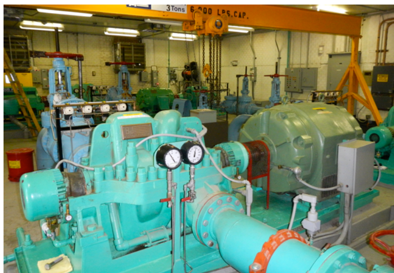
Luther Pass pump station is part of
