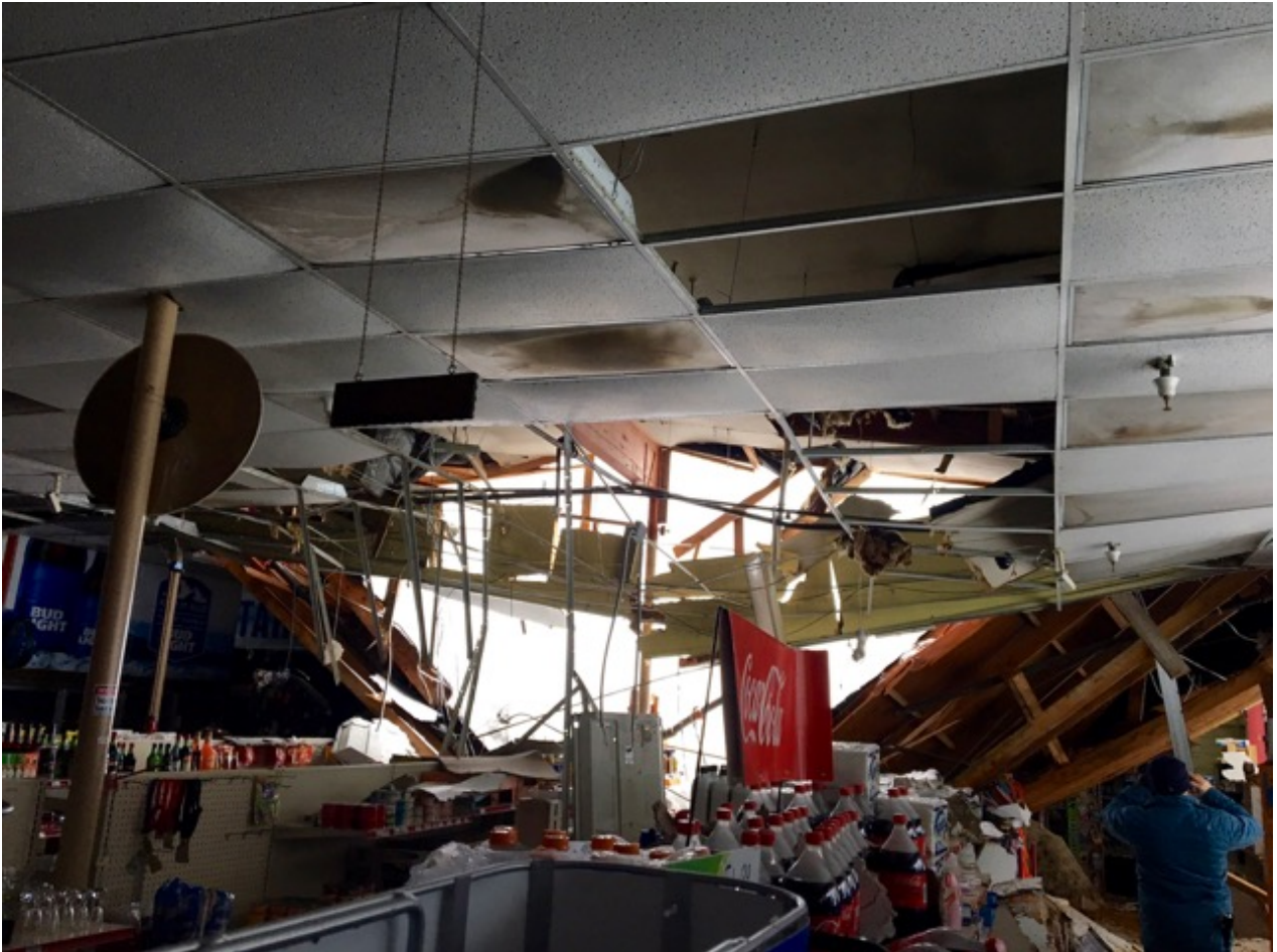
The liquor store could be a total loss after the roof collapsed Jan. 23. Photo/Provided
