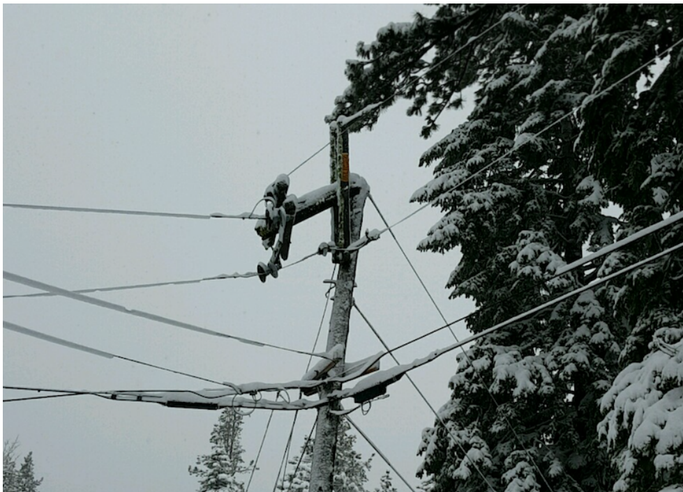
A broken pole this winter in the Ward Creek area took out power to Alpine Meadows ski resort and area residents. Photo/Liberty Utilities
