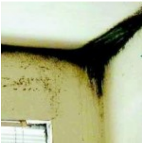
Mold at Bart's Apartments. Photo/South Lake Tahoe
