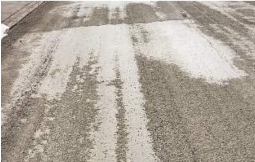
Tahoma roads disintegrated from a bad chip seal project. Photo/El Dorado County
