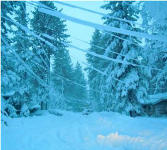
Sagging and downed power lines in Tahoe. Photo/LTN file
