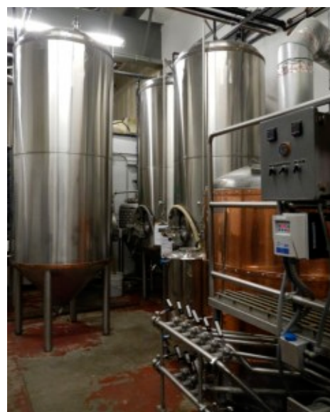
Tanks at the Truckee facility.
