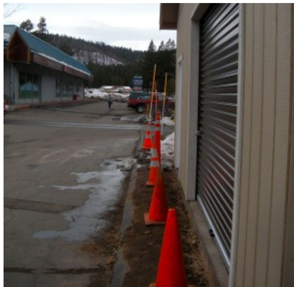
This structure houses remediation equipment to cleanup soil and groundwater contamination in South Lake Tahoe. Photo/LTN file
