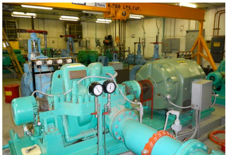
Luther Pass pump station is part of
