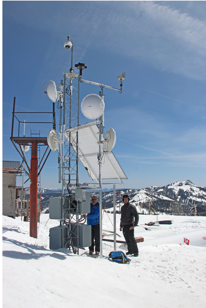
Nevada State Climatologist and Associate Professor Doug Boyle, and graduate student Paul Fremeau inspect one of three extreme weather stations at the crest of the Sierra Nevada at Sugar Bowl. Photo/UNR
