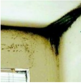
Mold at Bart's Apartments. Photo/South Lake Tahoe
