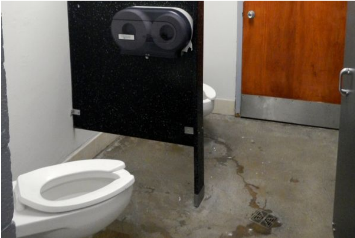
The South Lake Tahoe Recreation Center's men's bathroom lacks privacy. Photos/Kathryn Reed
