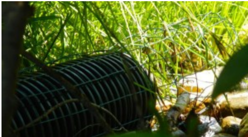
Pipes carry water through the beaver dam and wire keeps them from plugging up.
