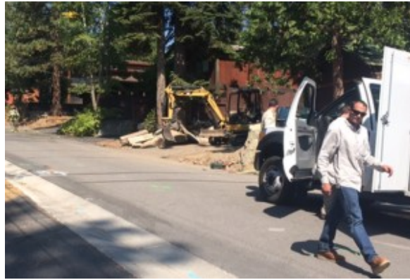
A backhoe struck a gas line in Tahoe City on Sept. 10. Photo/Provided
