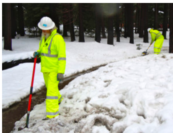
Caltrans crews in December 2010 work on a flooding issue along Highway 89.
