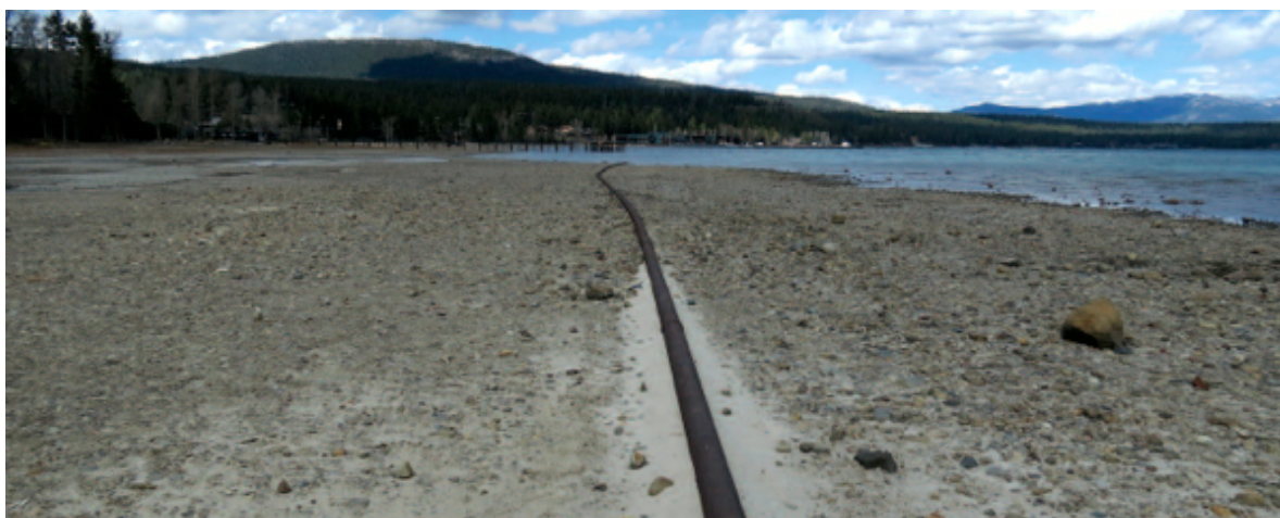
The beach with the exposed pipe.
