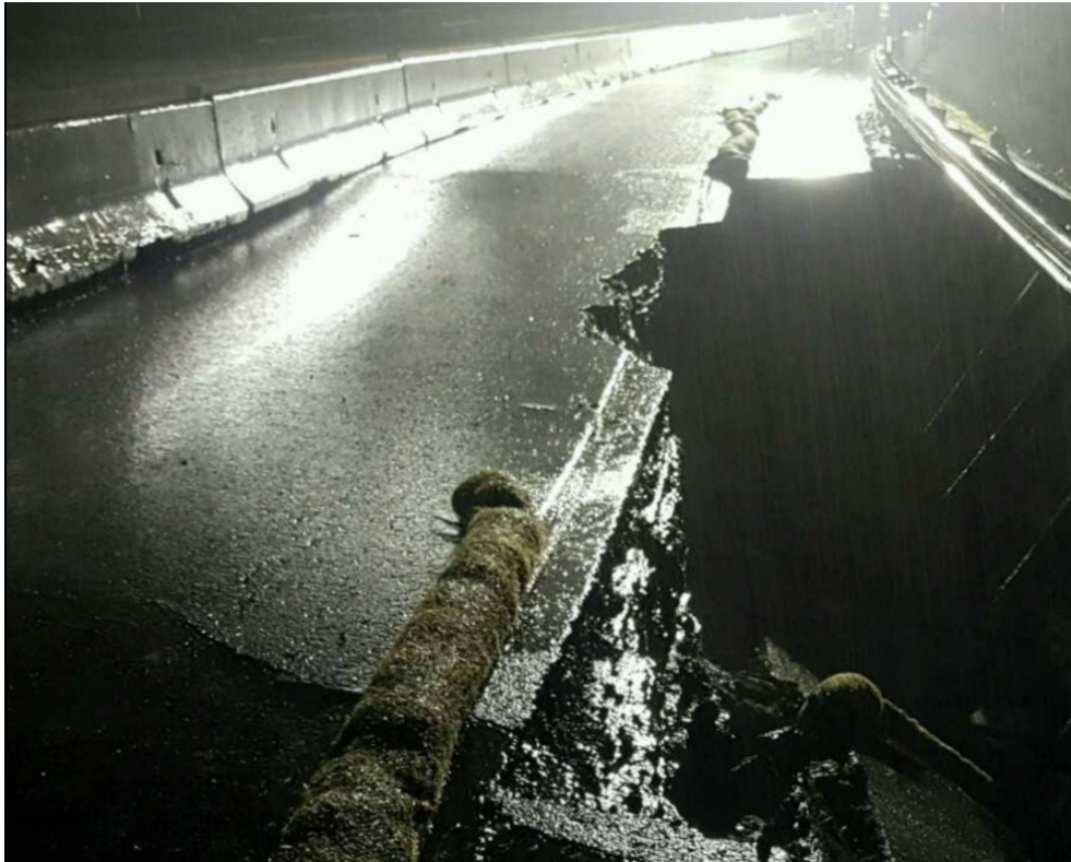
Highway 50 in the American River Canyon is washed out near Bridal Veil Falls. Photo/CHP
