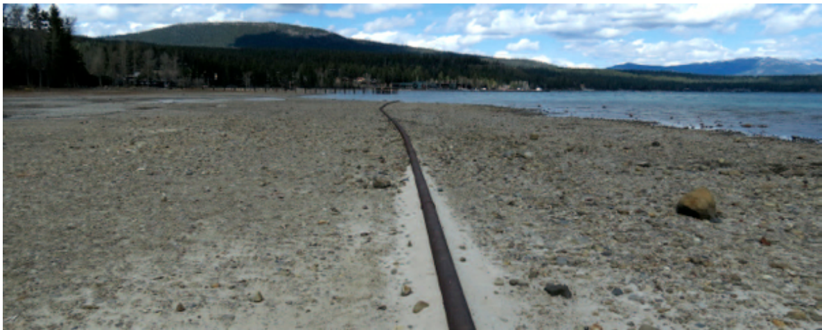
The beach with the exposed pipe.
