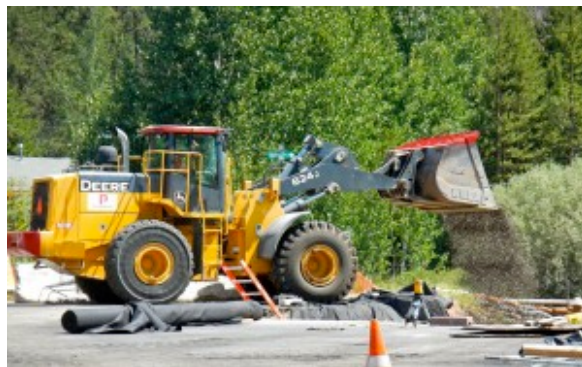
The Bijou erosion control project. Photo/LTN file
